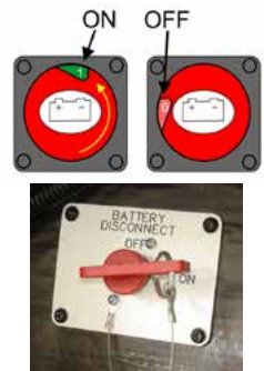
Battery Disconnect Switches
