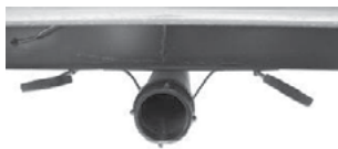
Black/Grey Tank Drain & Valves
